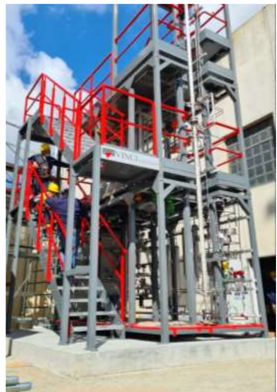
Vinci's E-Fuel pilot plant by CO 2 Utilization
